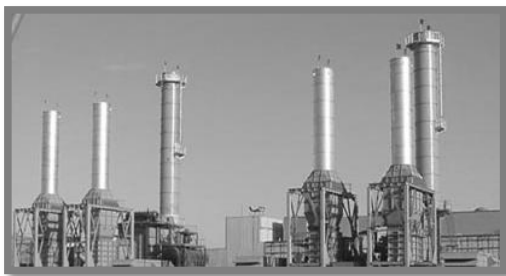
Gas-Fired Turbine Peaker Plant
