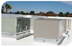
Ice-Ready™ Trane rooftop units and Ice Bear® energy storage units cut electric costs and demand.
